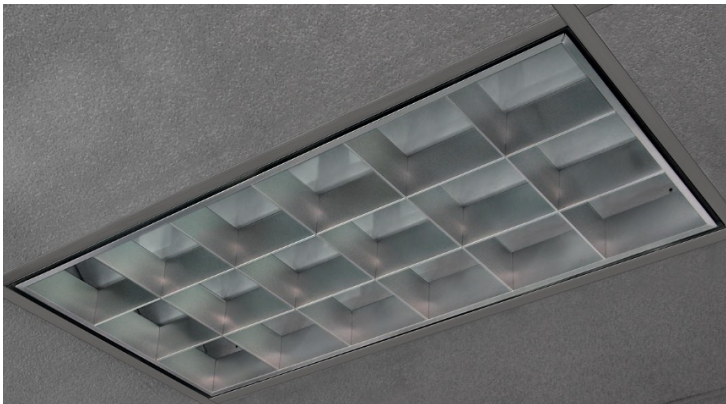
ORIGINAL FLUORESCENT LUMINAIRE
