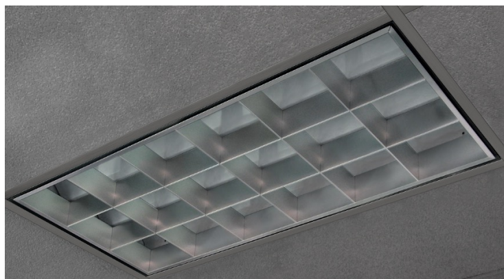
LUMINAIRE FLUORESCENT ORIGINAL
