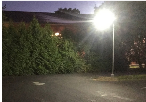
St. Paul's Church, MD - 6000 Lumens Install Height = 15 FT
