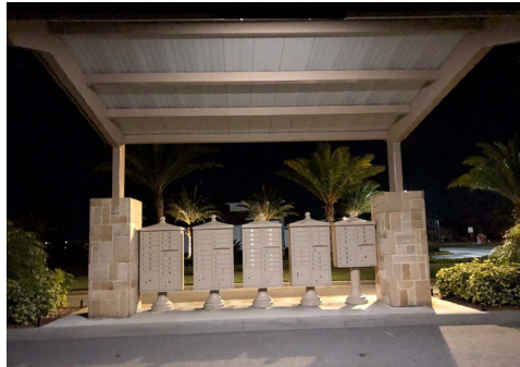
Valencia of Viera, FL - 2000 Lumens Install Height = 9-10 FT
